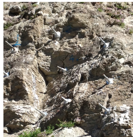
Ground anchors and rockfall protection.
