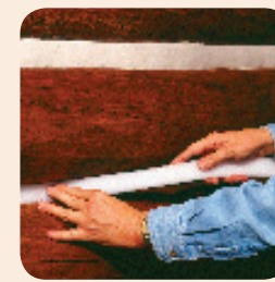
1. Start with logs that are stained with a coating compatible to Log Jam® and have properly installed backer material.
