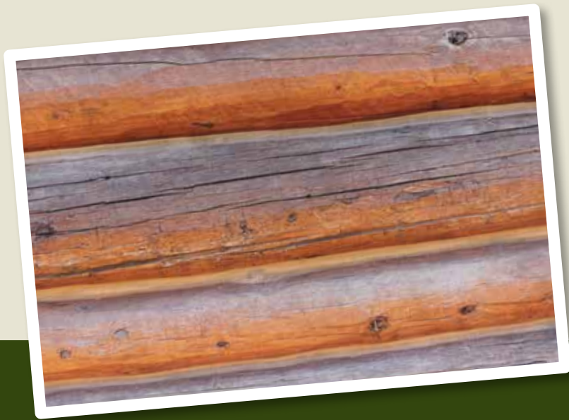
Deteriorated coatings like this need to be removed before re-staining.
