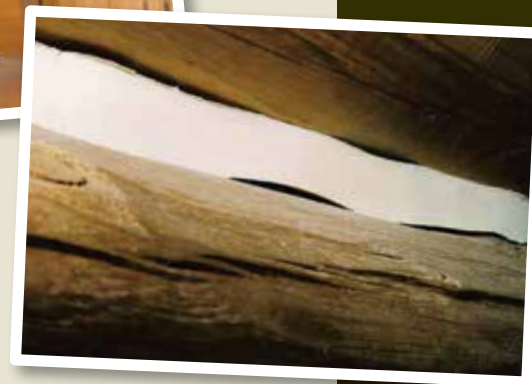
Adhesive failure of chinking
