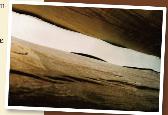
Adhesive failure of chinking
