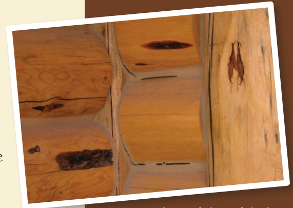
Cohesive failure of chinking
